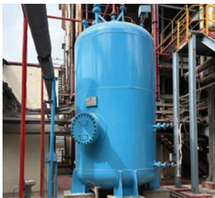
Buffer tank MTR Membrane unit at PVC Plant, Kota.
