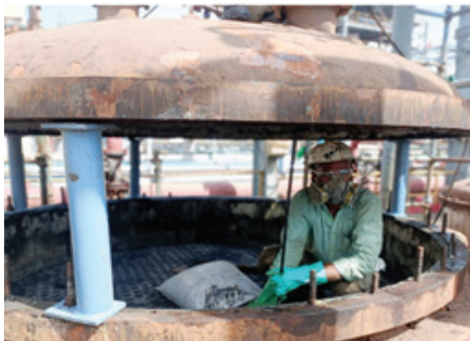
VC Reactor, PVC Plant.
